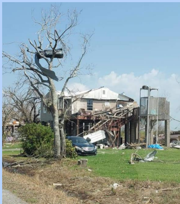
Farm damaged during Hurricane Ida, Louisiana, August 2021
